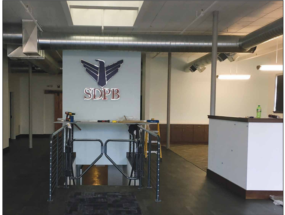
A work in progress, the interior of the Black Hills Bureau is taking shape.
