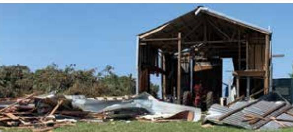
August 30 storm aftermath in southeast South Dakota.
